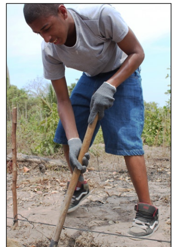
A Youth Ambassador in Mission (YAM) from the New York Annual Conference of the United Methodist Church digs a post hole Feb. 21 for a fence his team was helping construct in central Cambodia.
